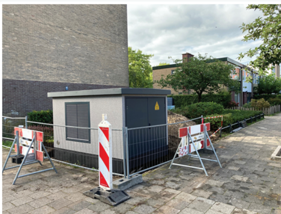
Figure 5: view of the transformer house next to which the BESS will be installed
